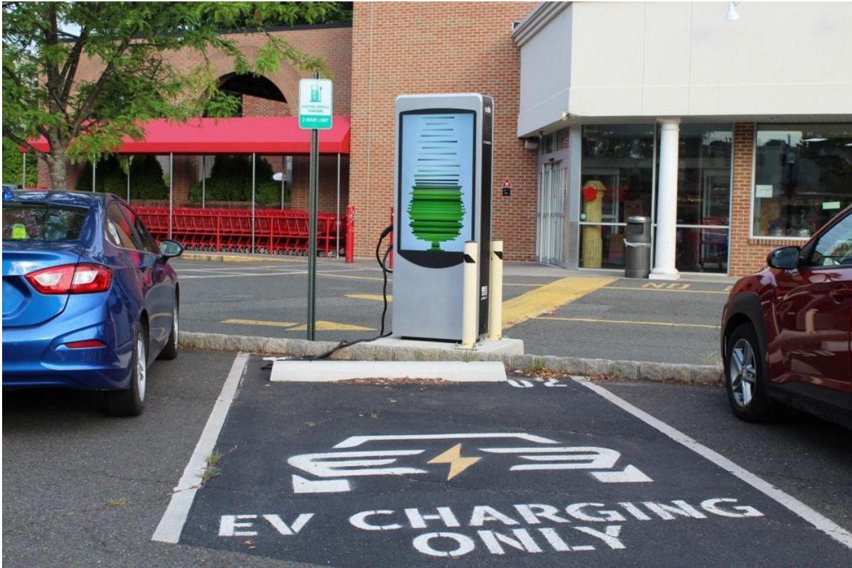
FIGURE II.1 CHARGING STATION IN WESTFIELD PUBLIC PARKING, AUGUST 8, 2022
